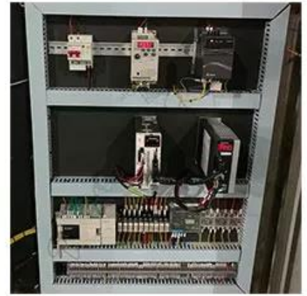
Machine Electrical Box
