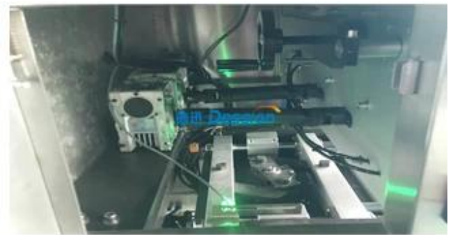
The power system
