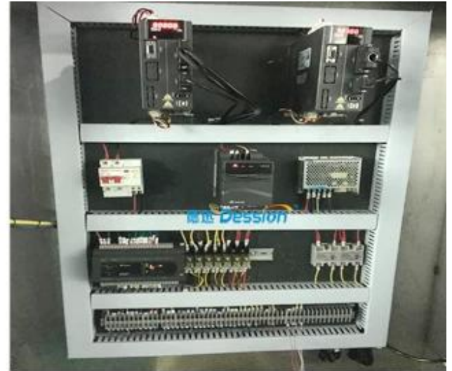
Electronic control components
