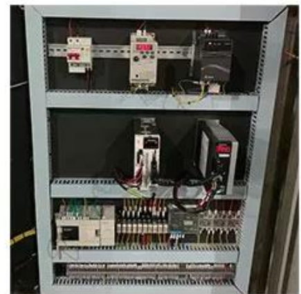
Machine Electrical Box
