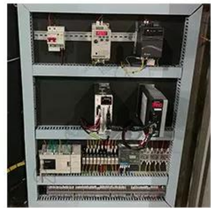
Machine Electrical Box
