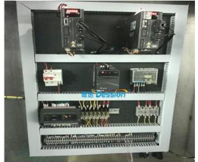
Electronic control components
