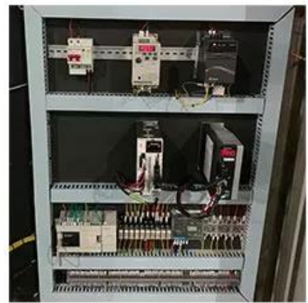
Machine Electrical Box
