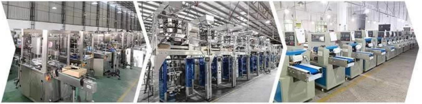
FILLING MACHINE WORKSHOP
