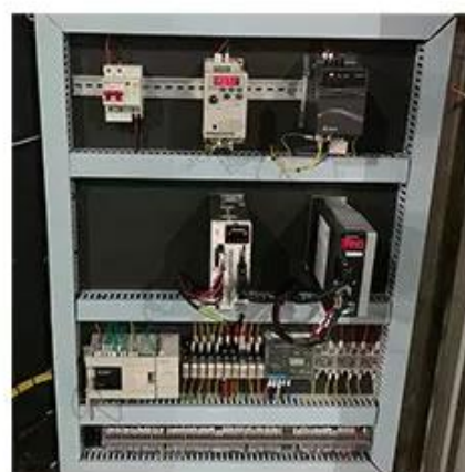
Machine Electrical Box
