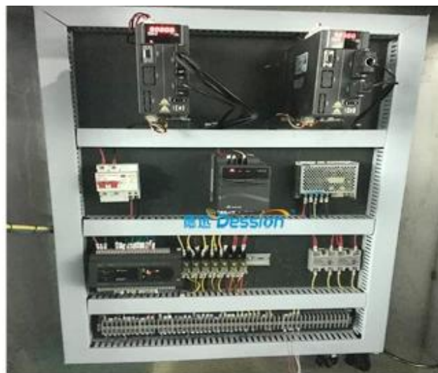
Electronic control components
