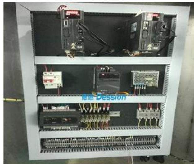
Electronic control components
