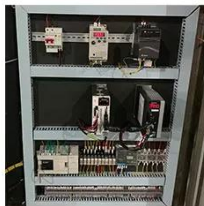
Machine Electrical Box
