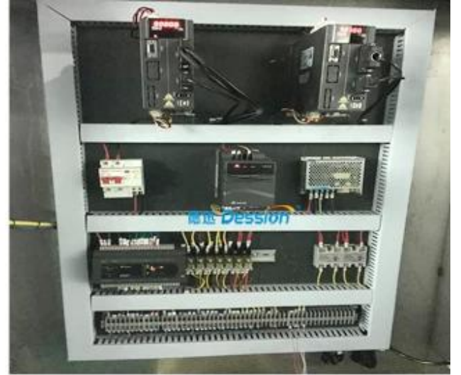
Electronic control components
