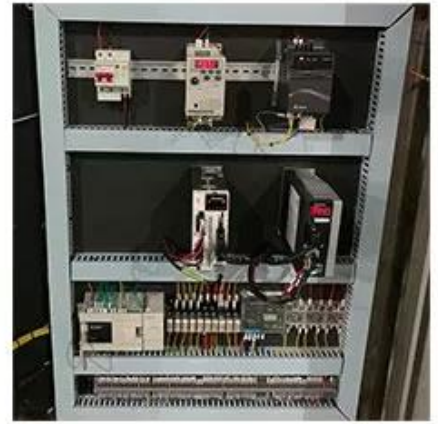
Machine Electrical Box
