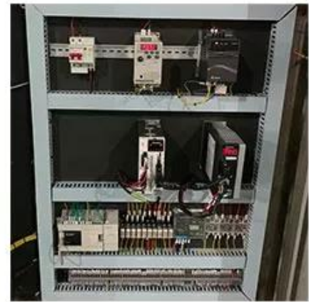
Machine Electrical Box
