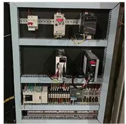
Machine Electrical Box
